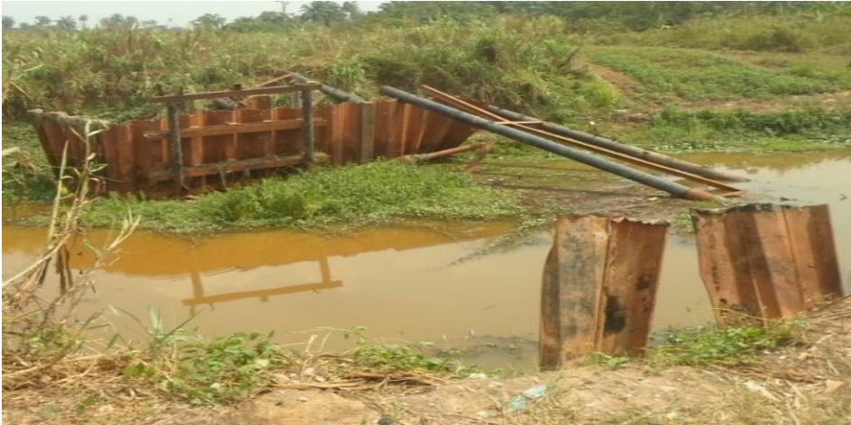
Plate1. Rusty and Dilapidated Iron Bridge in the Kolo Creek.
